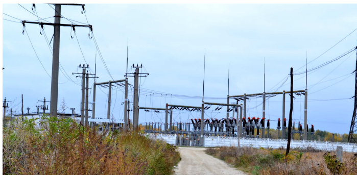
STATIE ELECTRICA - MARUNTISU
